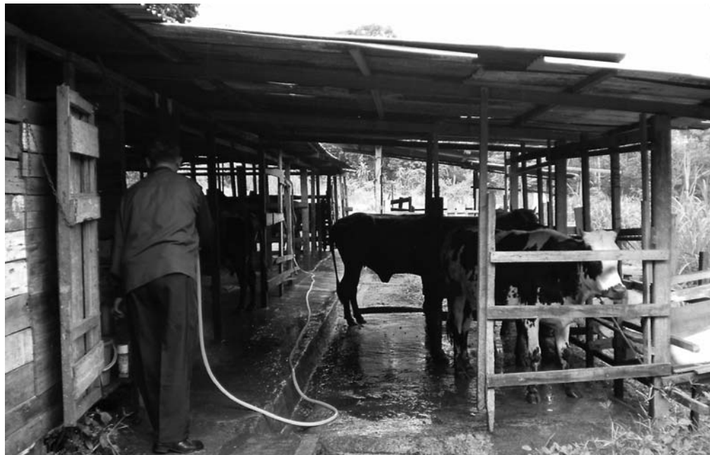
Figure 14.2 Sheds must be built for optimum cow comfort, not like this shed (Malaysia)
