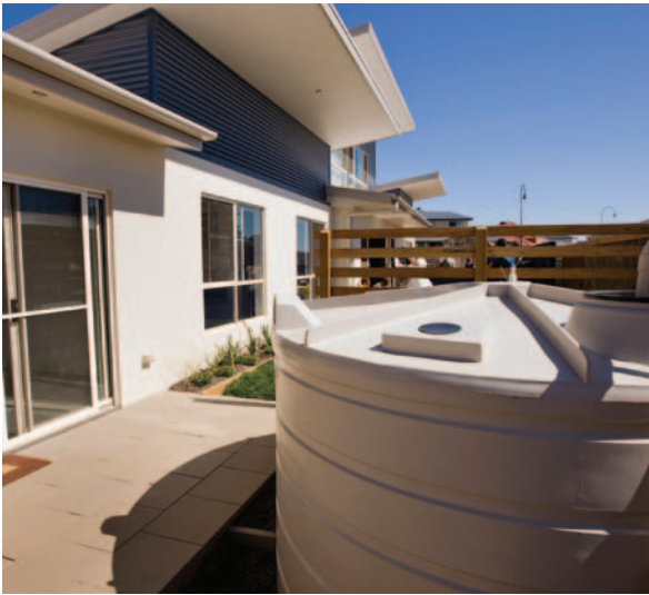
Domestic rainwater tank. Photo: CSIRO.
