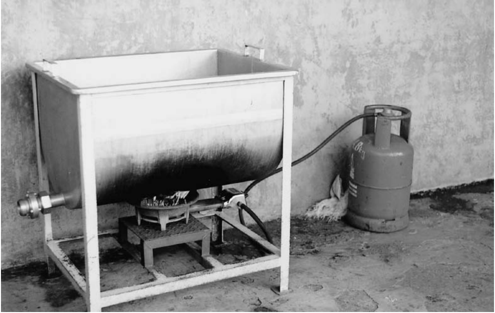
A simple gas water heater for ensuring hot water for cleaning empty milk cans at a milk collection centre (Indonesia).
