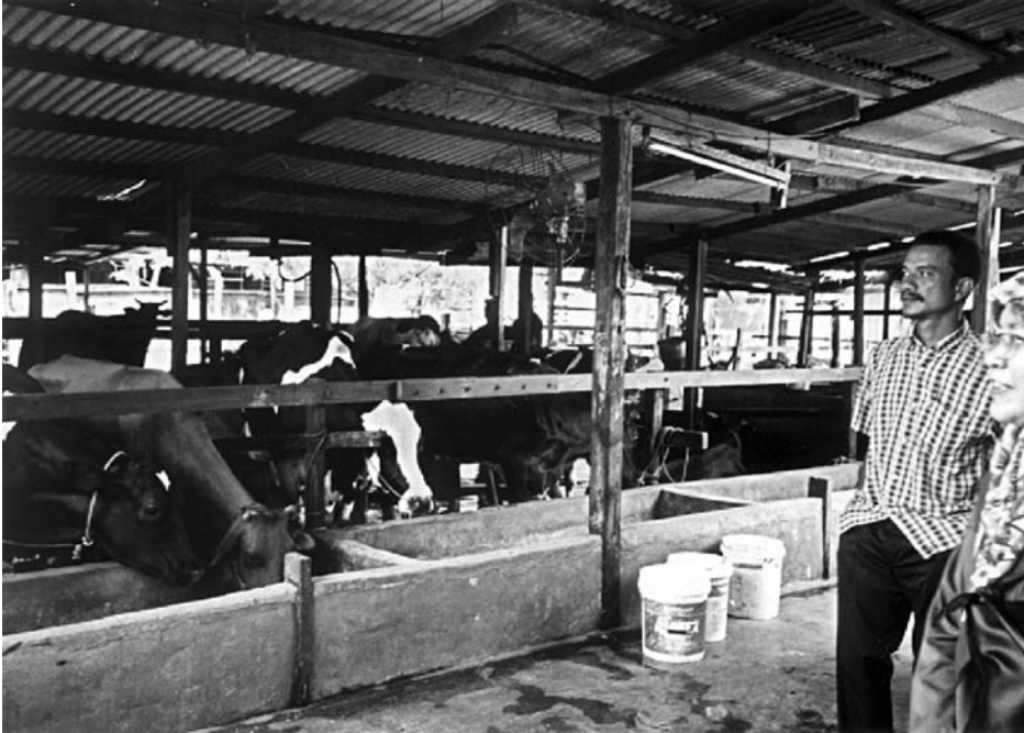
This shed is a converted piggery and clearly the roof is too low (Malaysia).
