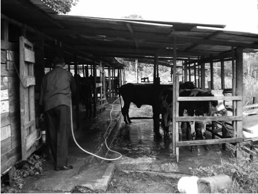
The roof in this shed is too low to allow adequate ventilation (Malaysia).
