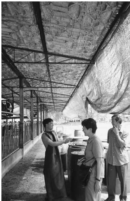
An effective insulation of a cow shed, using egg cartons (Banbeung, Thailand).
