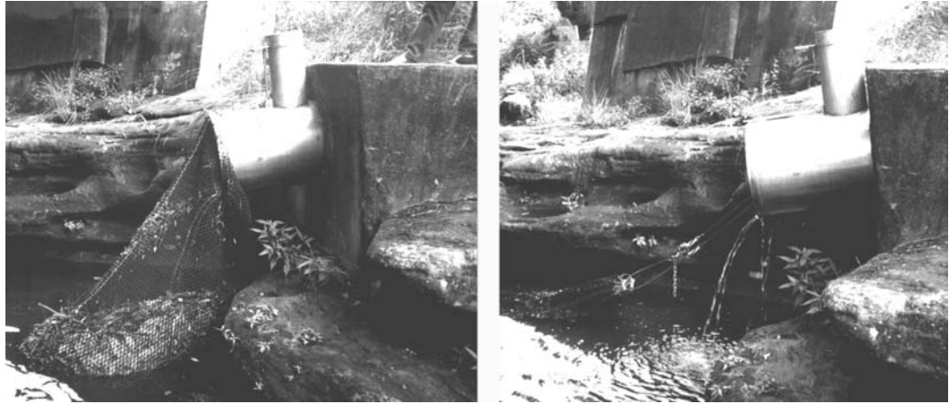
Figure 7.11 Release nets installed on a Sydney drain outlet.
