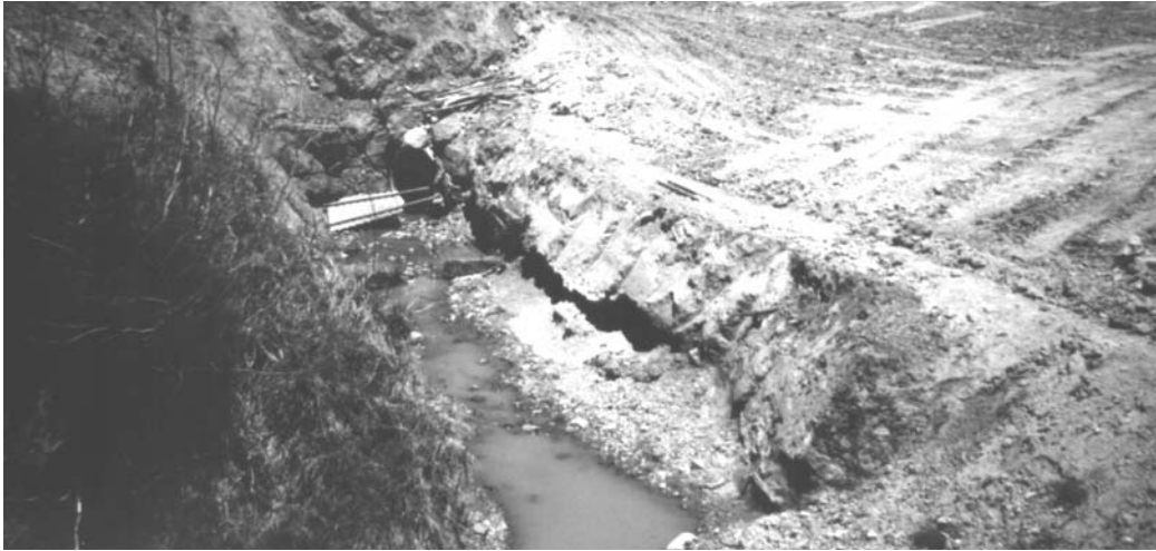
Figure 6.9 Exposed soils and unprotected drainage lines can erode readily.
